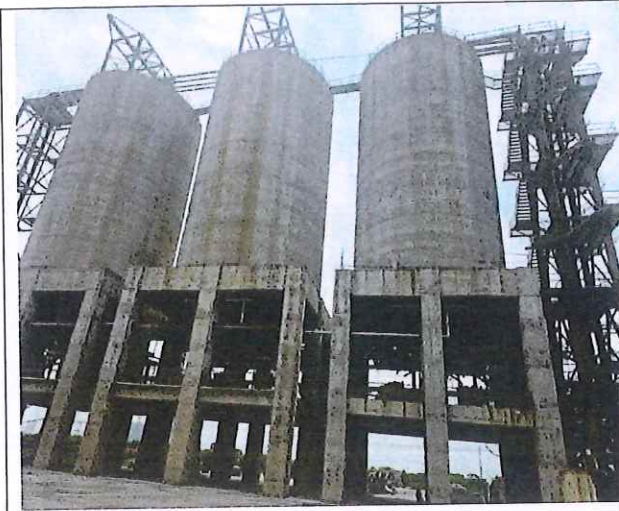
a) Silos provided for the storage of dry ash
